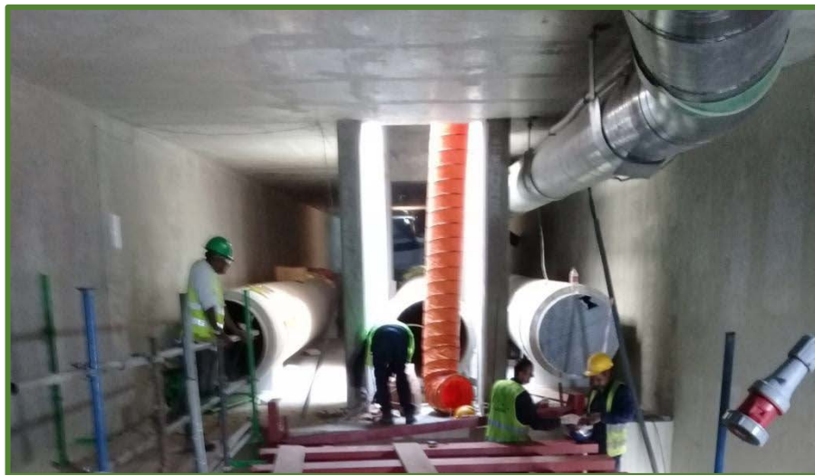
Pre-Insulated Pipes in Tunnel
